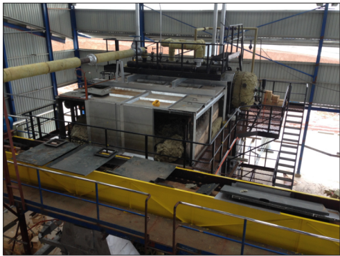
Assembling 20T/Hr boiler for steamproduction used to power a turbine and sterilise the full process.
