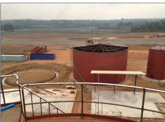
Preparation foundations and installation of a 2000T oil storage tank with steam coil.
