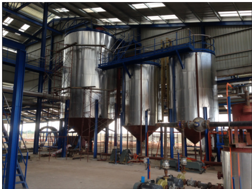
Insulating oil storage tanks.
