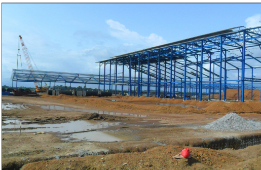
Groundworks, foundations and erection of steel structure. Steelstructure was prefabricated and imported from Malaysia.
